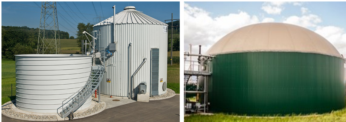
Abbildung 1-81 Thickener & anaerobic digester with integrated gas holder (Source: www.lipp-system.de ) and open digester with membrane covered gas-holder (Source: http://www.mifratris.de )
